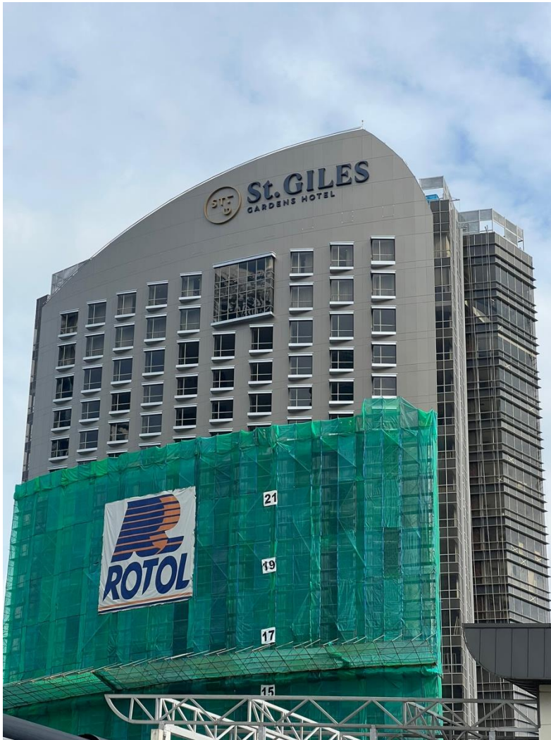
PVDF Aluminum Panels/ Cladding (Façade Refurbishment & Upgrading) St. Giles Gardens Hotel, KL
